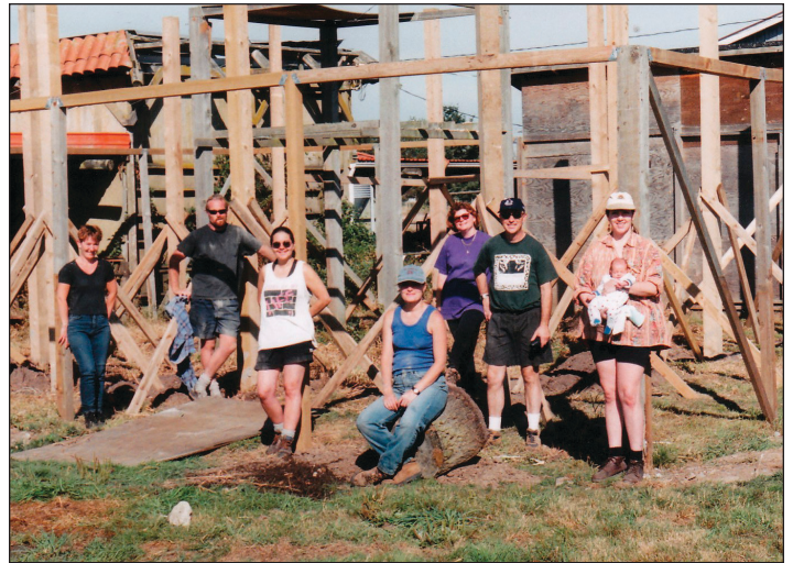
BOCSBC volunteers during construction of the South Surrey breeding facility. - Beer/Church photo
